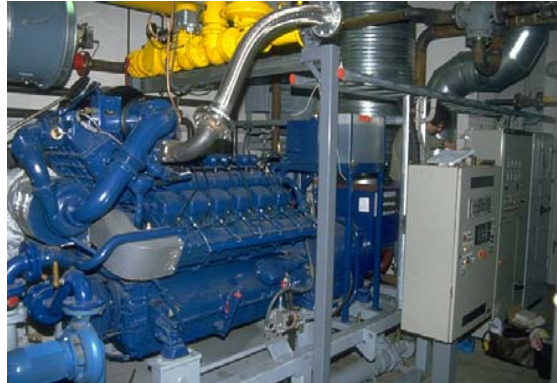
CHP - generation unit
